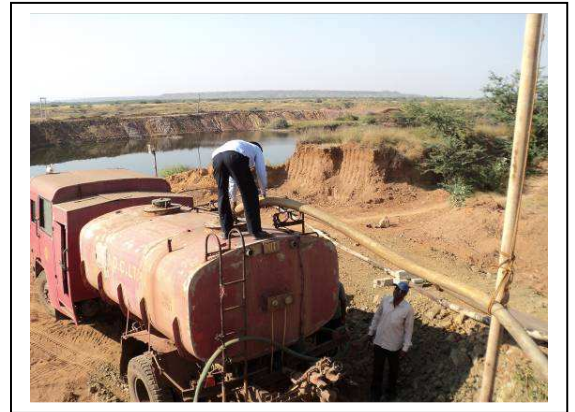
Alternatively tanker filling by gravity pipes to cater water requirements for plants
